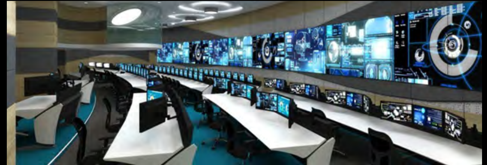
HITECH CONTROL ROOM
